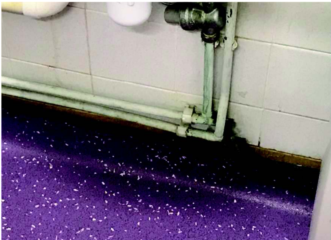
22 Dressed up skirting losing adhesion in accessible toilet
