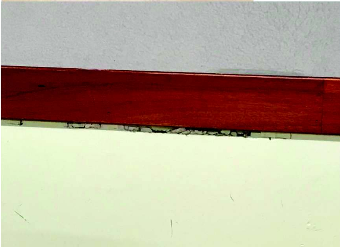
20 Damaged plaster below chair rail (rail is above height of tables)
