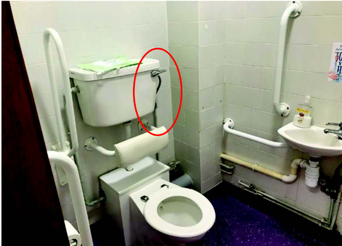
23 Flexi connectors at cisterns undersized causing delay in fill
