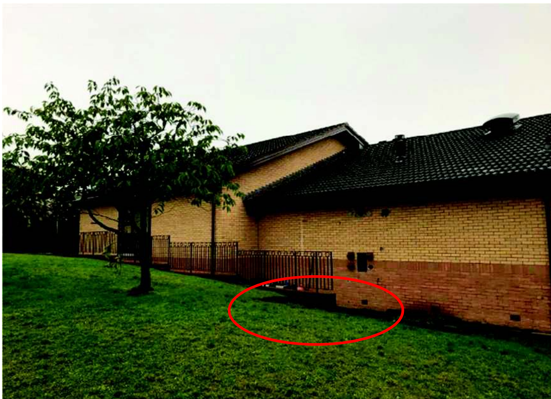
18 Area highlighted suffers from soil erosion at end of retaining wall. Consider installation of steps or re-dressing surface levels
