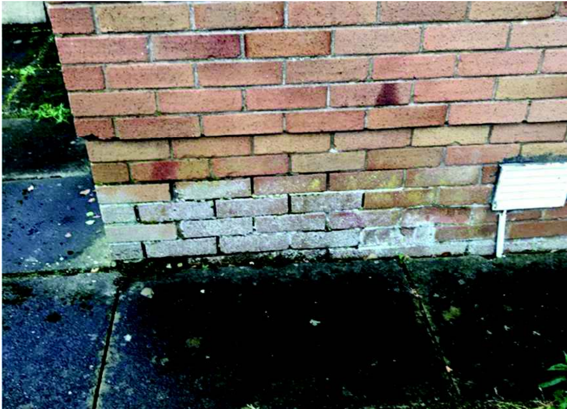
26 Efflorescence at corner at front - drainage appears blocked as gutter overflowing
