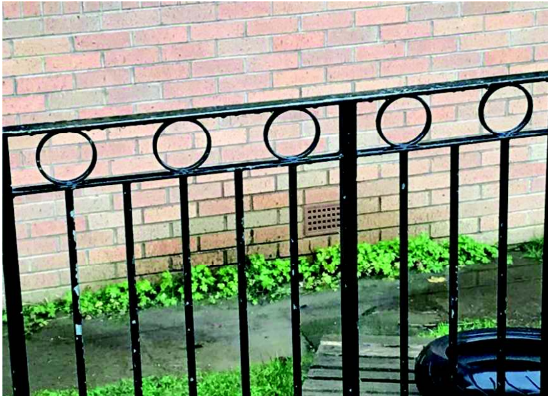
17 Check if ponding due to surface water run off from grass or from leak in gutter or below slabs
