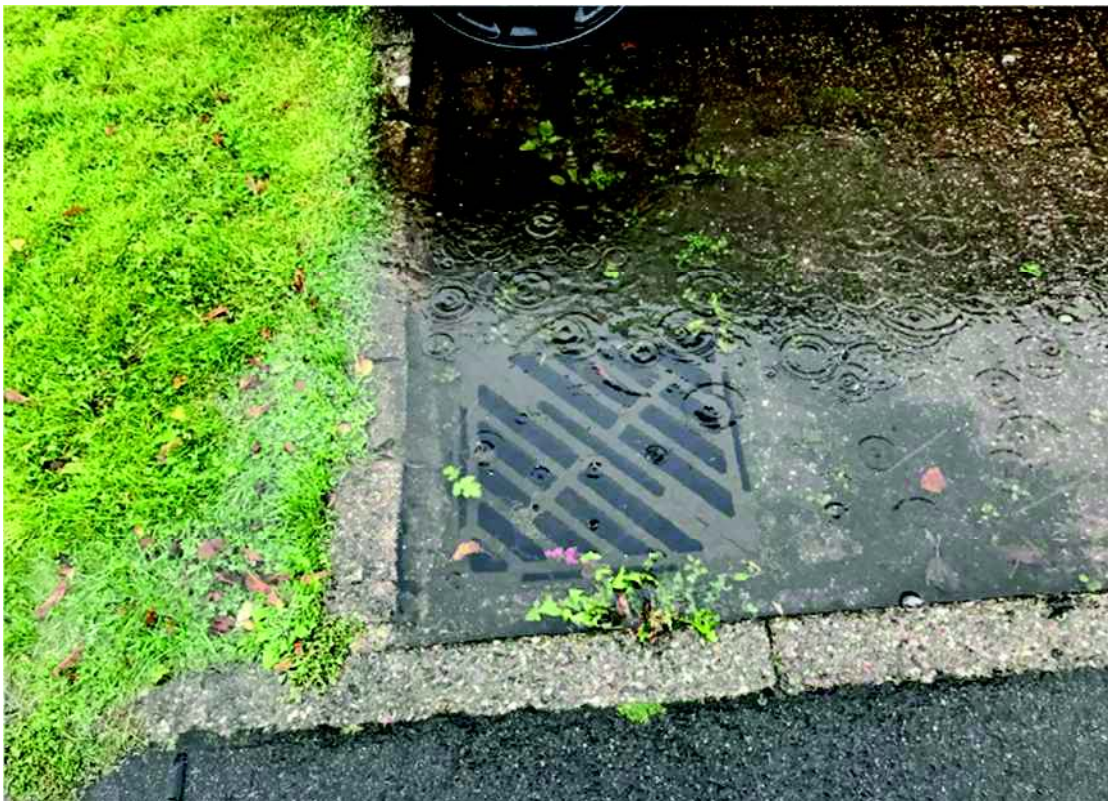
16 Car park gullies blocked
