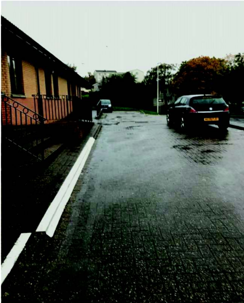
15 Monobloc sunk in various locations with trip hazards at manhole covers etc
