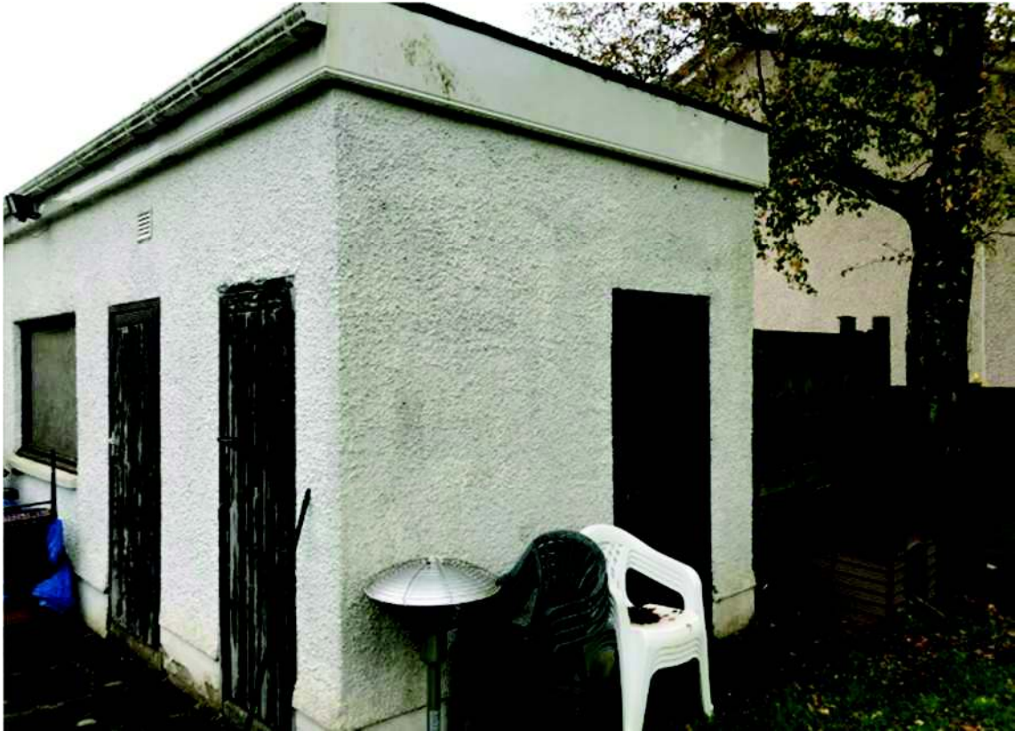
28 External woodwork to be redecorated
