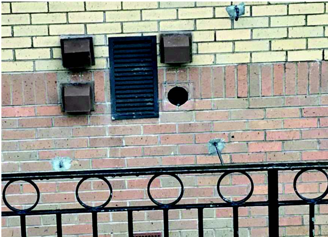
13 Missing vent cover
