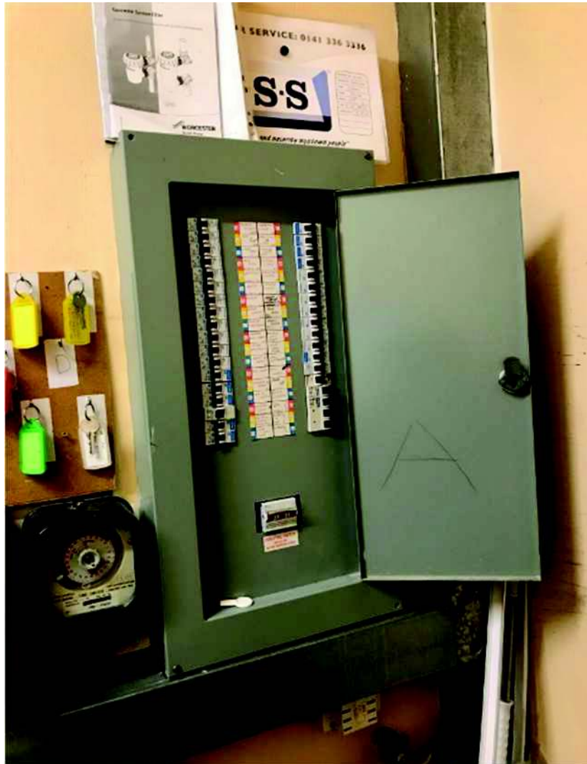
25 Main switchboard has no spare capacity
