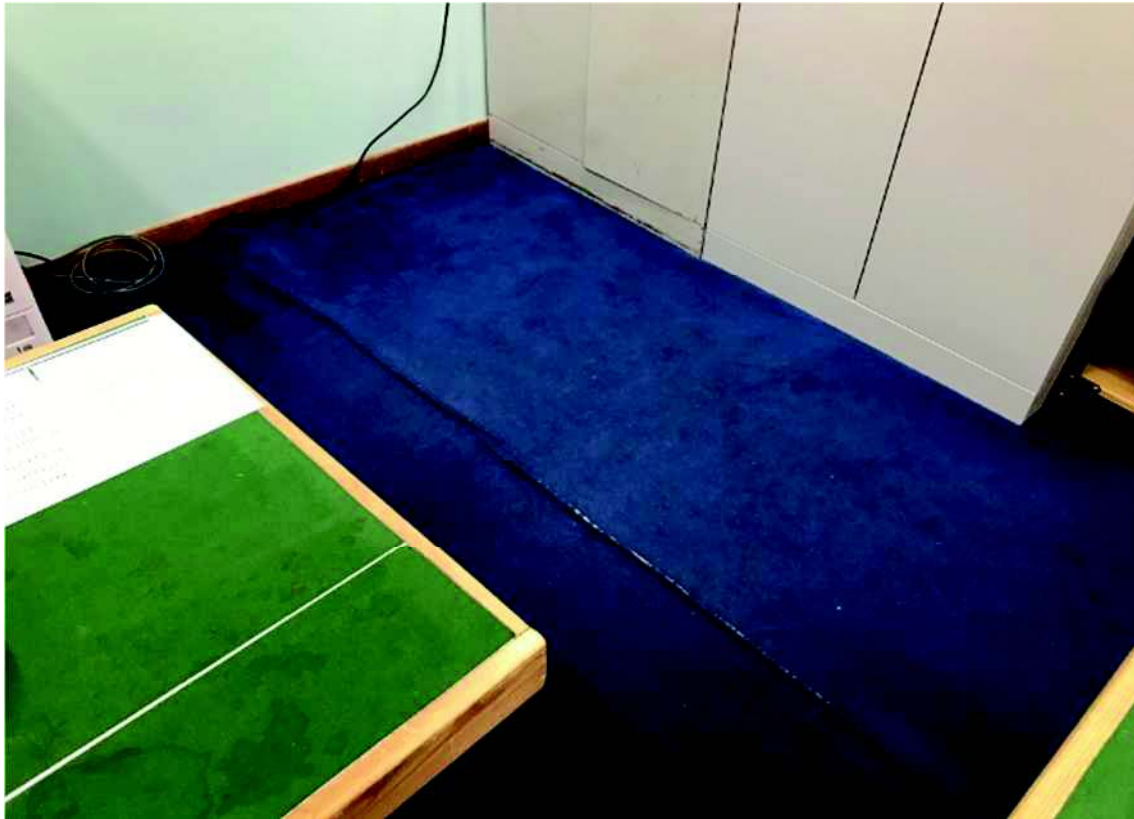
21 Crease in carpet in office
