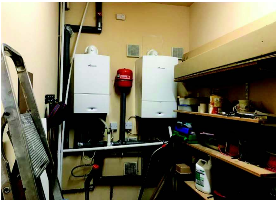
24 Boiler room - keep clear of combustible materials
