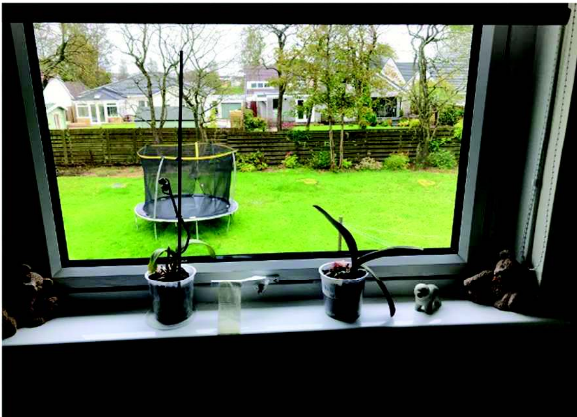
27 Window in upper hallway does not lock/close securely - taped closed at present. Replacement required
